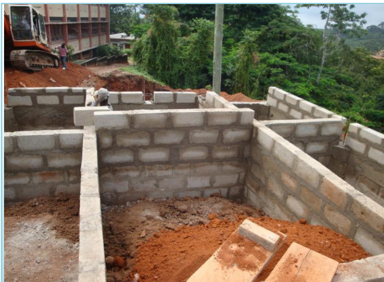
Mfantshipim waste management & power plant under construction. $20K to be funded by specified donations to PIE.
